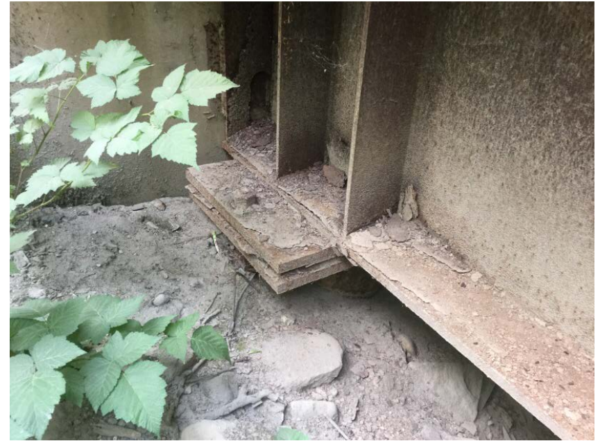
Minor steel delamination at left abutment
