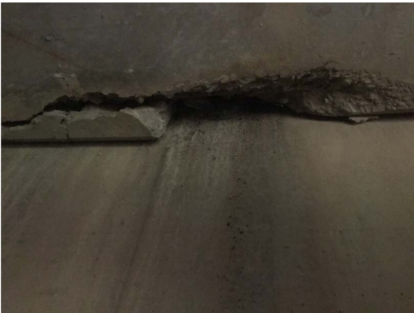
Damage to panel 1 on right approach
